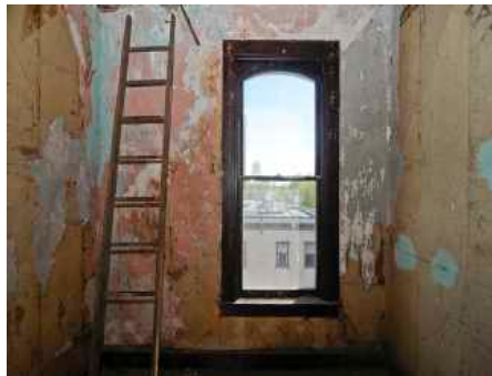
Pictures of windows before renovation
