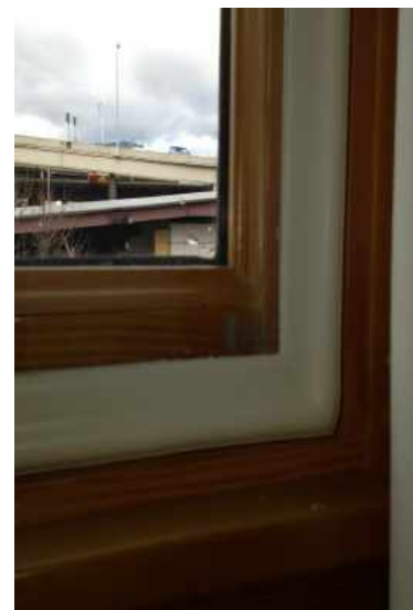
A window close-up after attachment installation. The attachment frame is in white and fits directly into the existing brown wooden frame.
