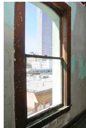
Pictures of windows before renovation
