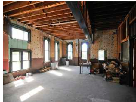
Pictures of windows before renovation
